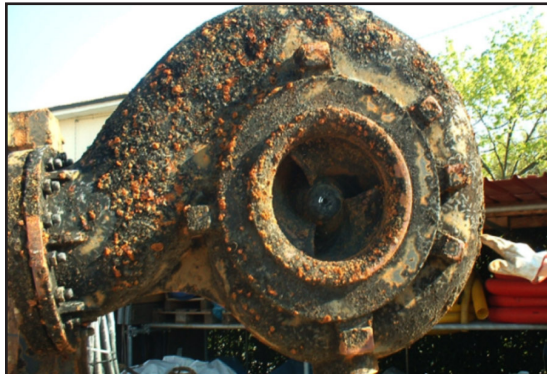
Eroded and corroded pump
