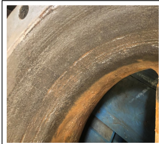
Severely damaged suction bell before being repaired with ARC 858.
