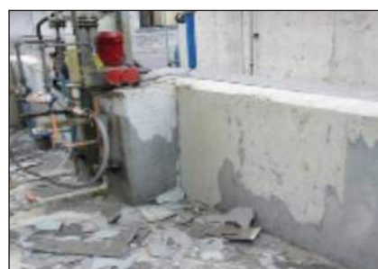
Failed coating of secondary containment area after spills.
