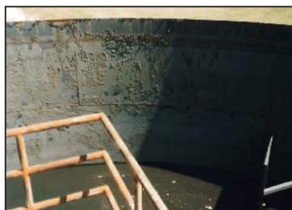
Failed coal tar epoxy coating
