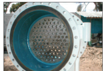
After ARC 858 has rebuilt corroded areas two coats of ARC SD4i is applied.
