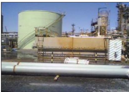
Basin in petrochemical complex
